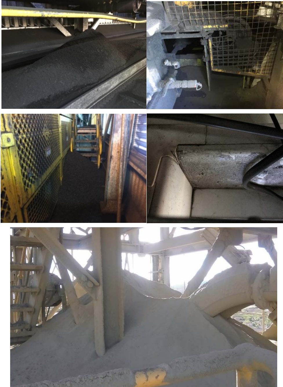
Figure 9 Images of dust build-up in coal-fired power stations in Queensland
