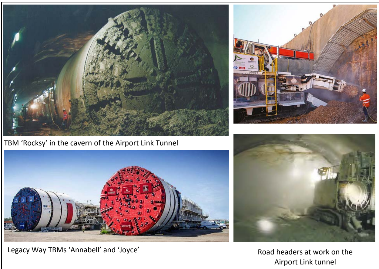
Figure 10 Tunnel boring machines and road headers used in the construction of Airport Link and Legacy Way
