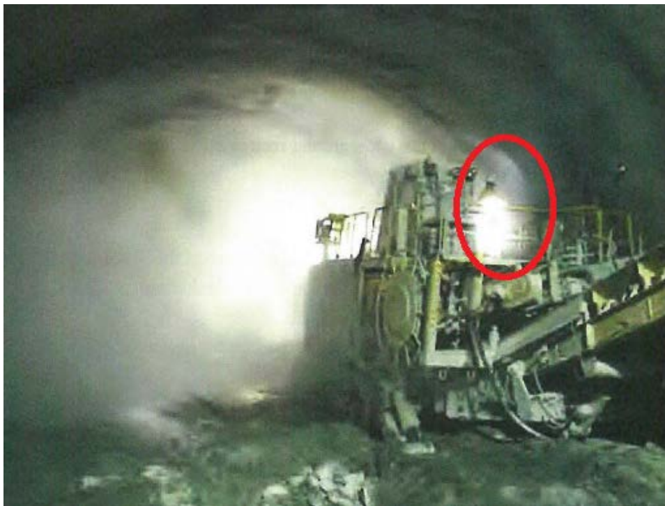
Image 2 Road header operator out of sealed cabin in close proximity to the dust cloud, Airport Link construction
