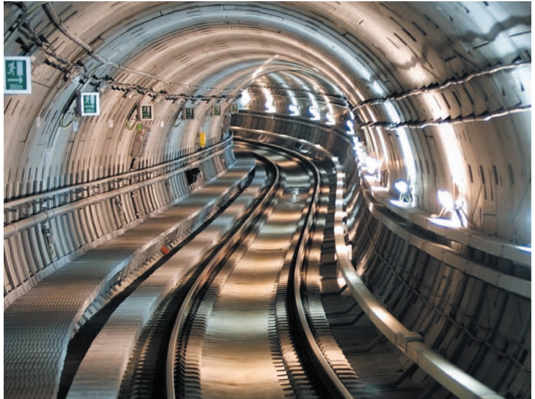
Commissioned tunnel infrastructure
